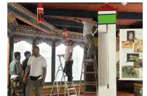
Above: New lighting systems were installed during the relocation project
