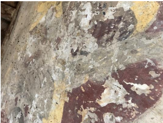
The spots on this medieval wall painting are little bat droppings sticking to the painted plaster
