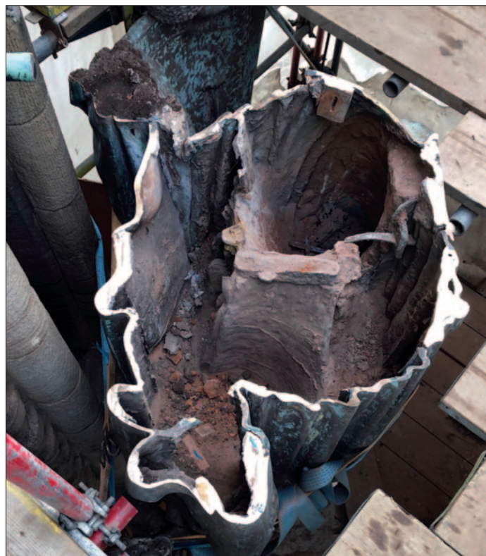
The hips and legs remaining. The slot for the locating cotter can be seen on the far side, the crotch joint is in the centre and the sand filling can be seen below
