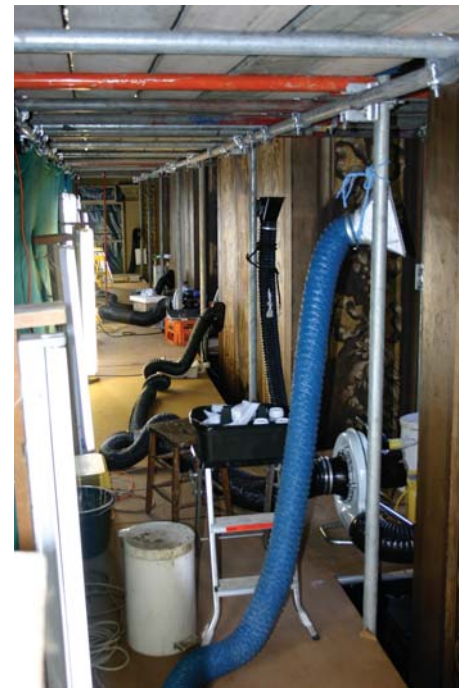
Portable extraction system
