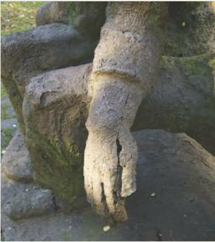
A split along a construction seam line
