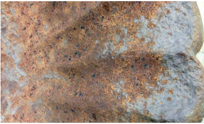
New corrosion erupting after dry blast cleaning. Note the black spots
