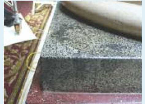
Detail of Scagliola repair to the base of a column in the Grand Hall
