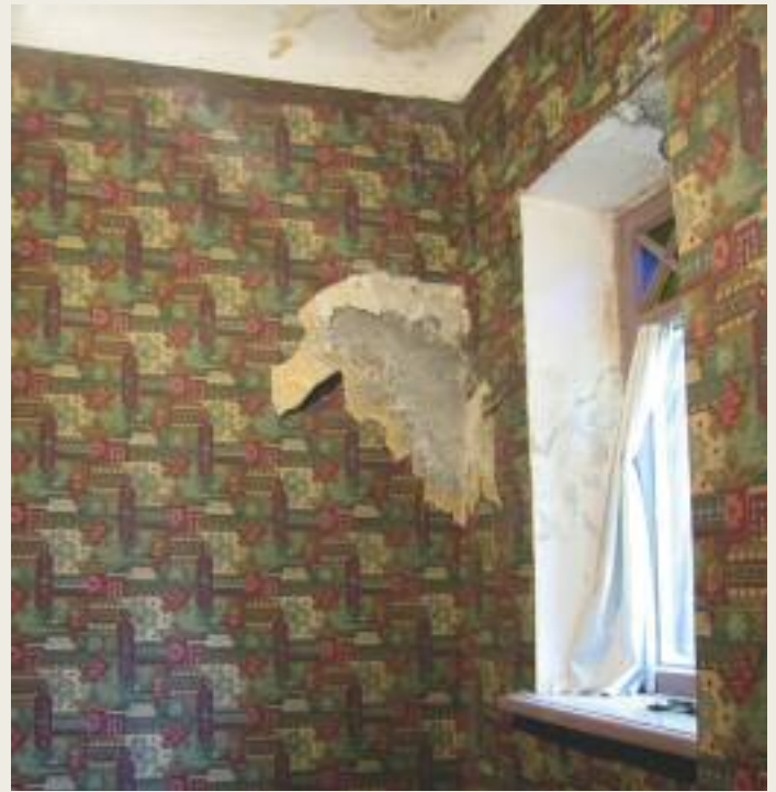
Damaged wallpaper. This has since been repaired but only as a stopgap measure, since there is no proper heating in the house and the mould is likely to return.
