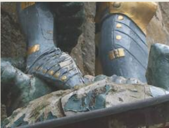
The flaking paint on St George's right foot
