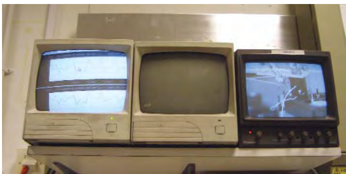
Cameras viewing inside radiation room
