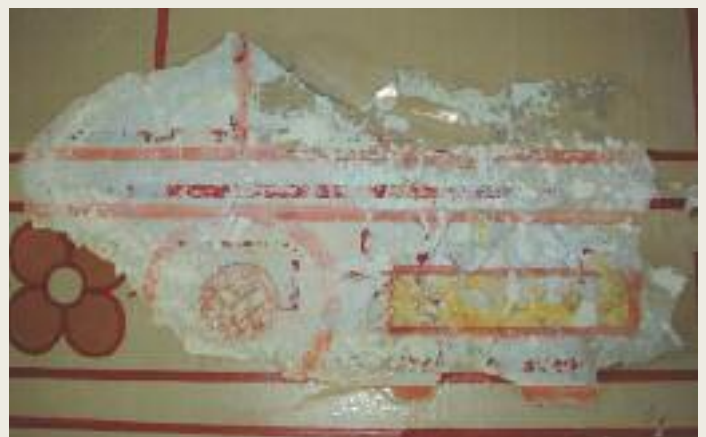
Remnants of earlier decoration revealed in damaged areas
