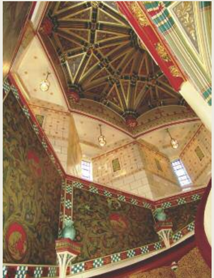
The Octagonal staircase with efflorescence damage before conservation
