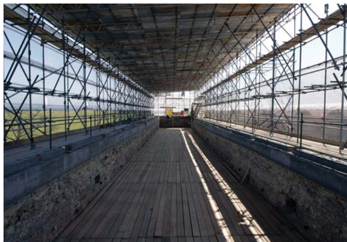
A view of building work to the Knole studio at roof level
