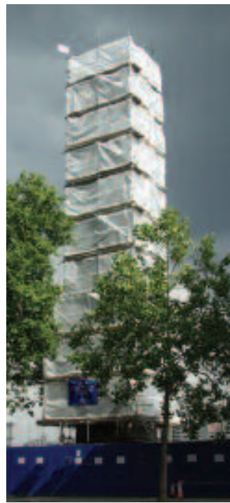
Full scaffold erected, with monoflex sheeting. Hoarding with warning signs 'No public access'
