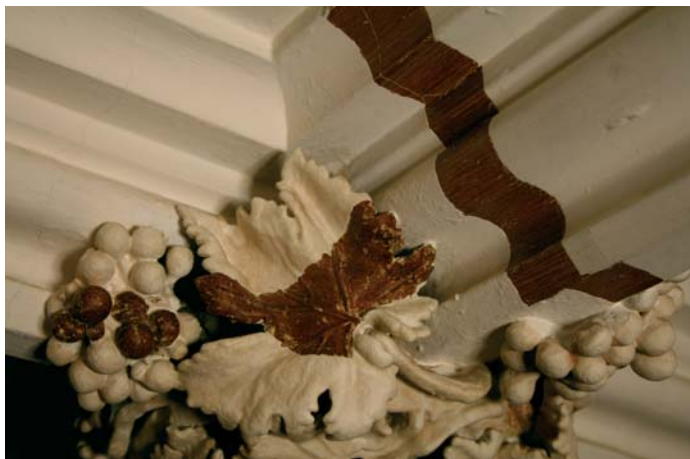
Dining Room original graining revealed on moulding
