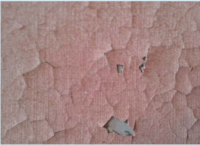
Detail of flaking paint
