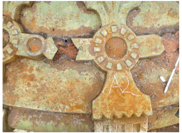
Frost heave fracture
